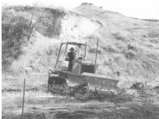
Moving earth to make way for the new Lewis & Clark Native Plant Garden at the Idaho Botanical Garden in Boise.
